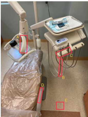
Figure 1: Sampling locations within the dental operatory assessed to evaluate the effectiveness of an electrostatically applied US-EPA N List effervescent disinfectant, (2,153 ppm: 5 minutes contact time), sodium dichloroisocyanurate ((NADCC) / C3Cl2N3NaO3 (US-EPA Reg. No. 71847-6-91524)).
